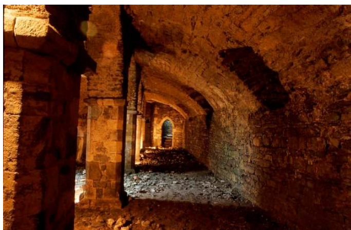
Interior of 13th century undercroft looking south to doorway to stone spiral stair
